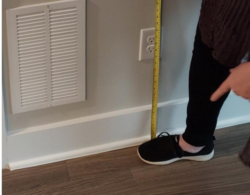
Figure 6: Less than 15” to Operable Outlet
