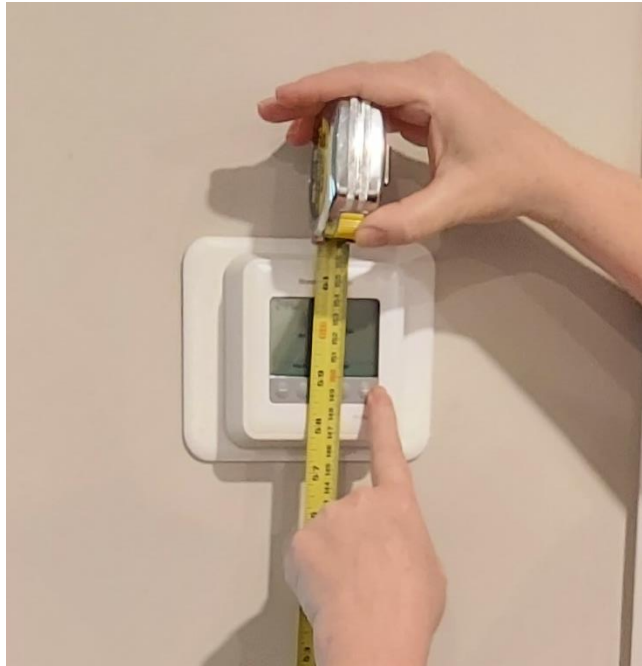
Figure 5: Appx. 59" to Operable Component of Thermostat
