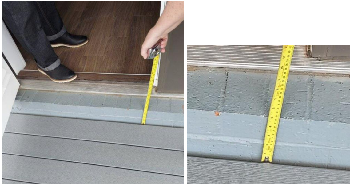
Figure 4 (with zoomed-in image): Exterior 5" Step at Unit Balcony
