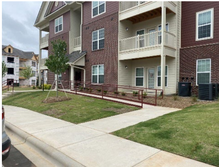
Figure 12: The accessible route from Building 105 to the Community Center does not contain a curb cut.
