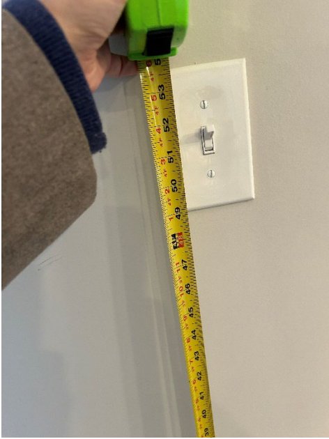
Figure 32: Operable part of light switch at Revere at River Landing above 48 inches
