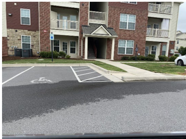
Figure 30: The access aisles for disabled parking spaces at Revere at Tega Cay are too narrow because they do not “have an adjacent access aisle that is 60 inches wide.” Design Manual at 2.20.
