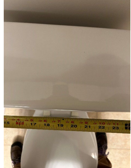
Figure 35: Distance between adjacent wall and centerline of toilet at Addison Park exceeds 18 inches.
