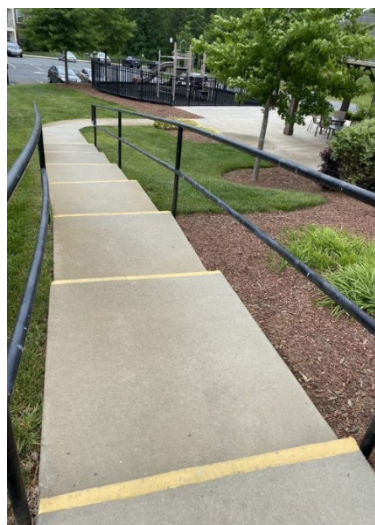
Figure 11: Stairs along the route from the Community Center and Pool to the playground at Revere at Lake Wylie.
