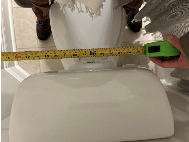
Figure 34: Distance between adjacent wall and centerline of toilet at Revere at River Landing exceeds 18 inches.
