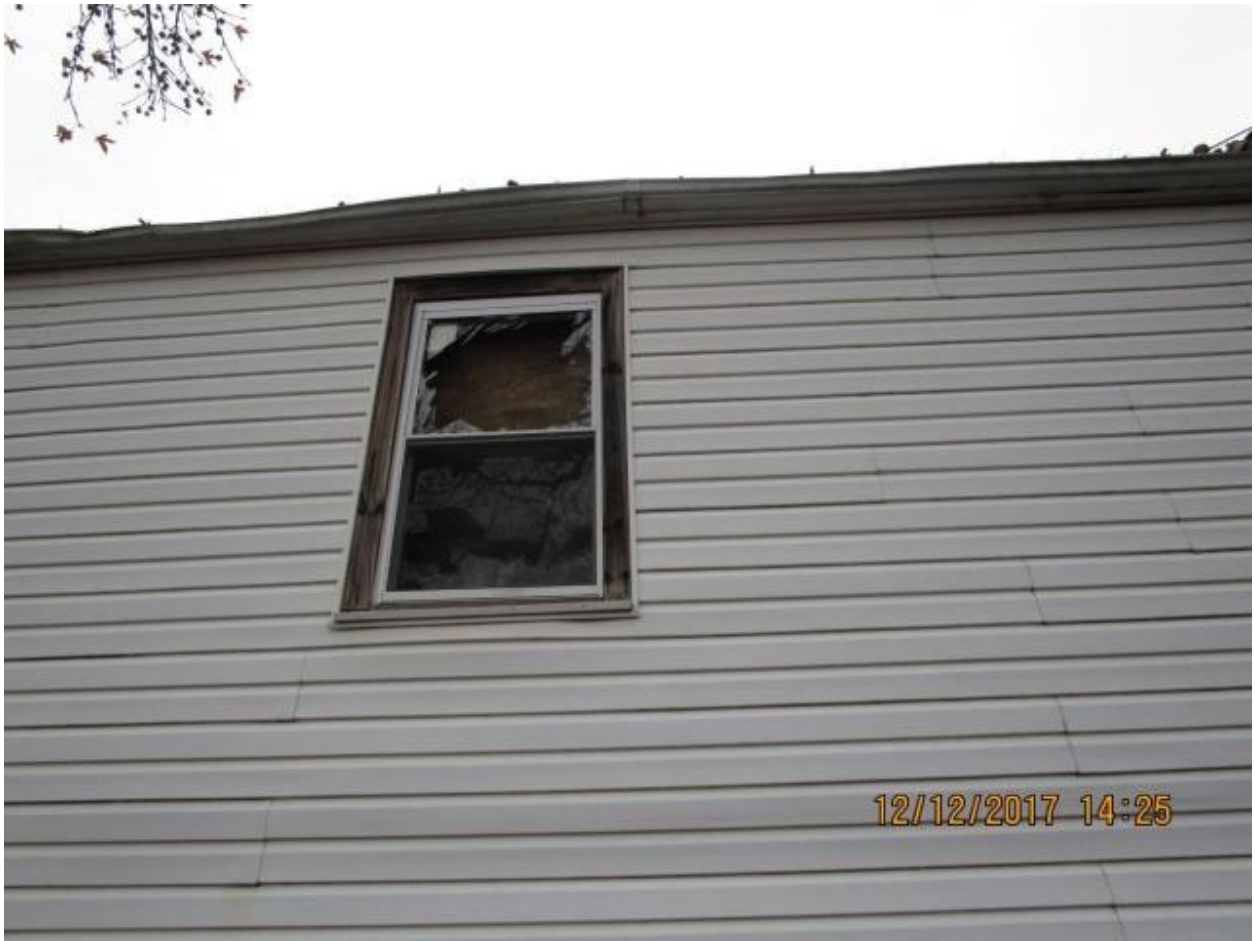
Capitol Heights, MD – Broken window
