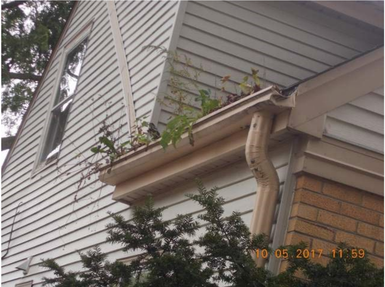
Milwaukee, WI – Obstructed gutters
